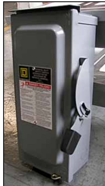
PICTURE 9: Power Disconnect Switch
