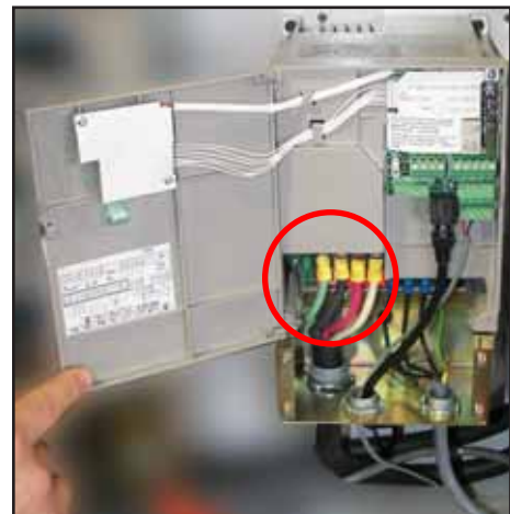
PICTURE 6: 3-Phase Inverter Wiring
