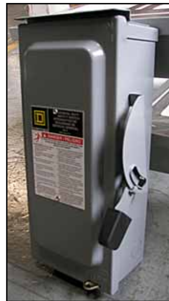
PICTURE 4: Power Disconnect Switch
