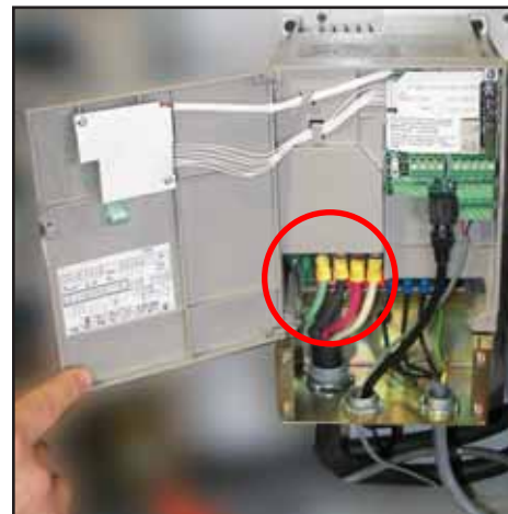
PICTURE 6: 3-Phase Inverter Wiring
