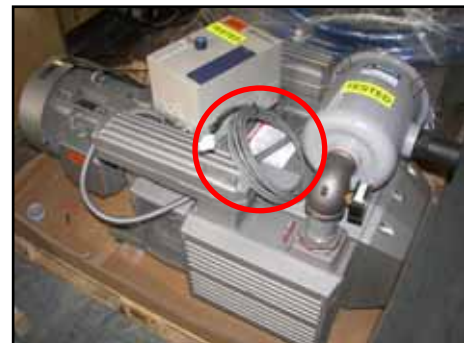
PICTURE 10: 3-Phase Wired Pump
